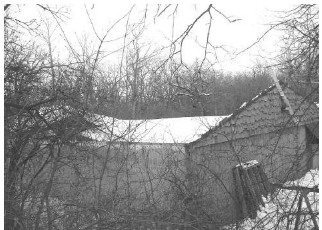
The collapsed barn – January 2005
